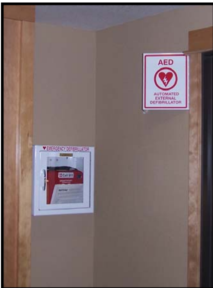
The Automated External Defibrillator (AED) is located in the lobby of the Cliff Lodge. Sign up for trainings on how to use the AED and for CPR and first aid classes.
